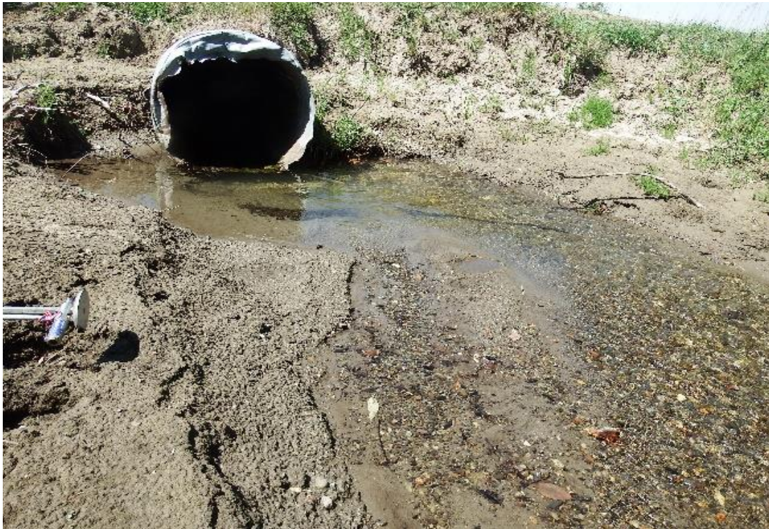
Figure 6-4. Culvert and siltation in Jones Creek about two miles downstream of the South Valley Road crossing.
