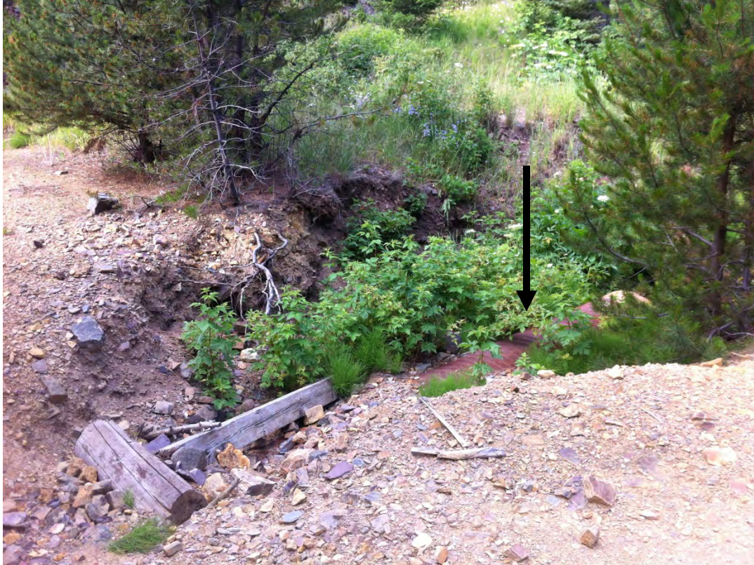
Figure 3-1. Failing culvert (pipe indicated by the black arrow) in the Sandbar Creek watershed
