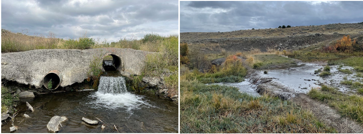
A. B. Figure 1. A) Looking upstream at the dam in 2022 before beavers blocked the second culvert. Erosion underneath the cement structure is evident. B) In 2023 beavers blocked the culvert and the stream began forming a new channel to the north of the existing channel and culvert.
