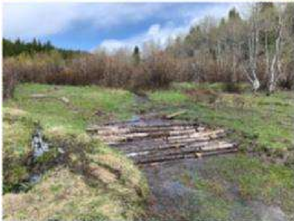
Check dam structures installed during low flow improve natural storage and floodplain connectivity.
