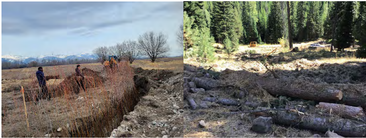
Figure 4: A willow trench is installed to address the absence of woody riparian vegetation and increase floodplain roughness (left- photo by Leah Swartz). A former user-built road that was de-compacted, covered with logs and slash, reseeded with native grass seed, and then covered with straw mulch (right).
