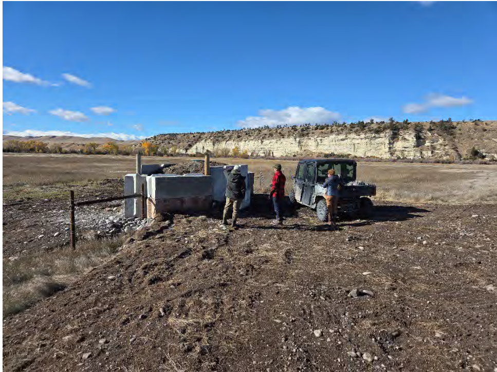
Figure 7: One of the new stock tanks designed by Max Jones. The tanks are designed to be self-filling and resistant to freezing.
