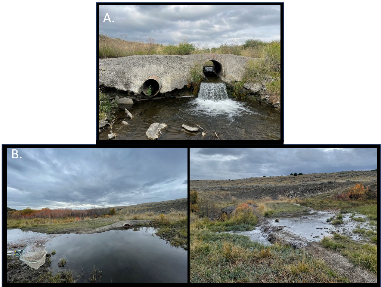
Figure 1. A) Looking upstream at the dam in 2022. Erosion underneath the cement structure is evident. B) In 2023 the stream began forming a new channel to the north of the existing channel and culvert.
