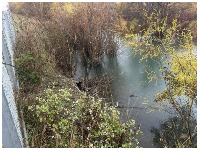
Figure 6. Culvert view with damming materials inside. West Dry Creek Road.
