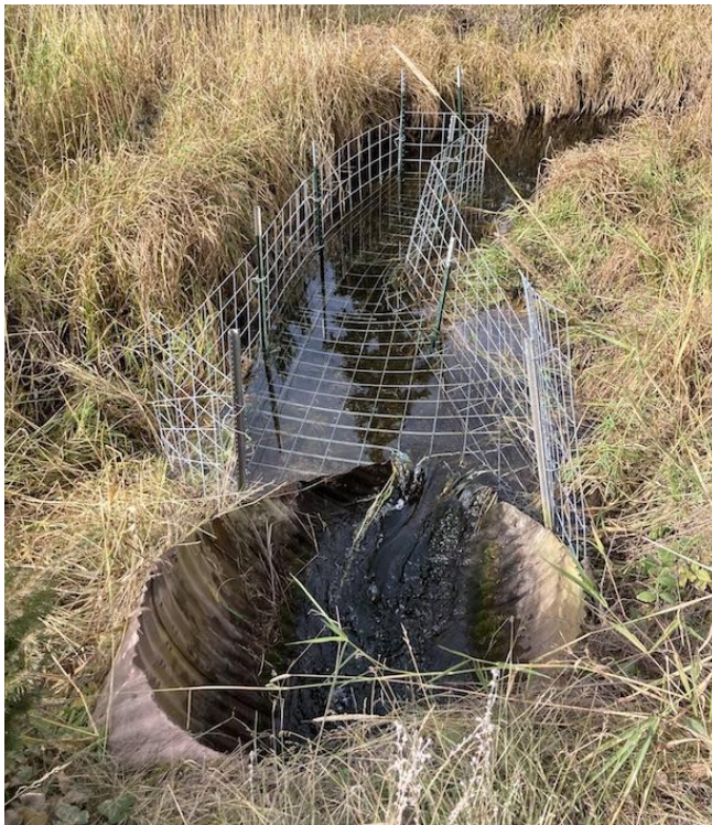
Figure 8. Exclusion fence to prevent culvert plugging on a Lolo National Forest Access Road, Seeley Lake, within the Clearwater WRP.
