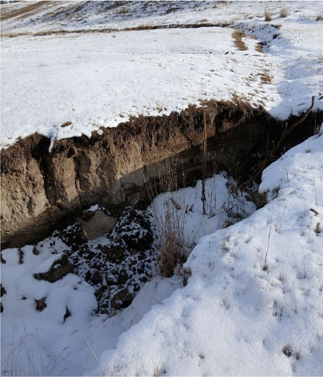
Site Photo 4, Unit 2: Headcutting at ditch outlet into Cameron Creek.
