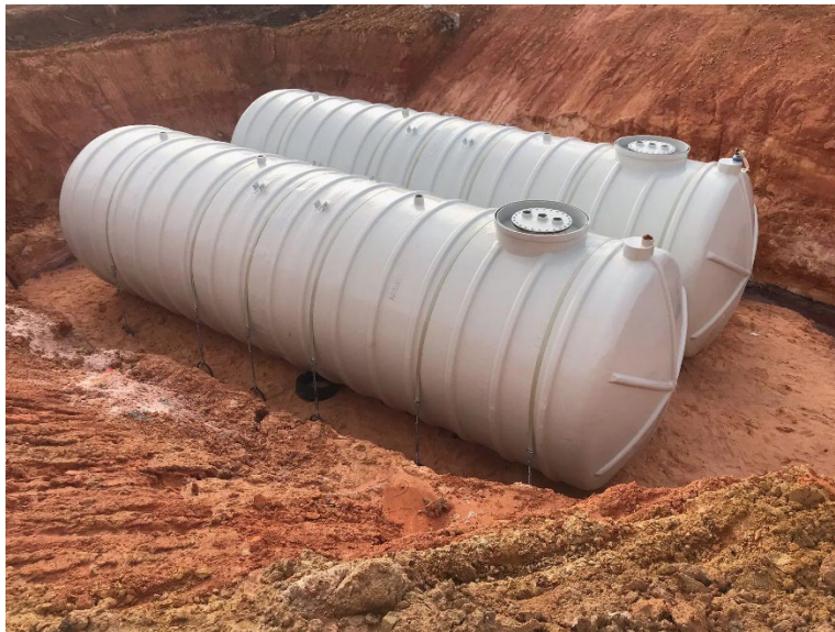
Figure 3: Underground Water Tanks
