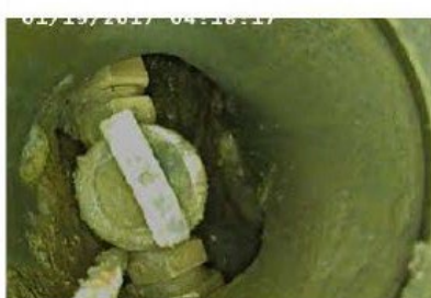
Non-Lead Service Line
