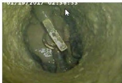
Lead Service Line
