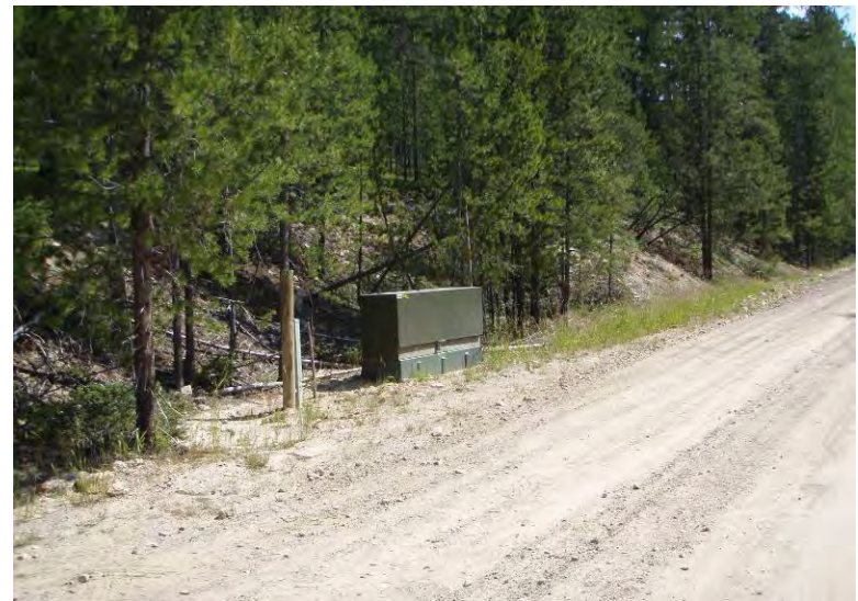
Photo 28: Power junction box on east side of Mike Horse Creek Road (looking SE).
