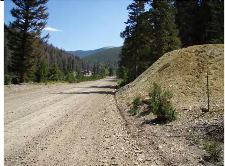
Photo 2: Waste/Tailings Pile below collapsed Mary P adit along Mike Horse Creek Road (looking easterly).
