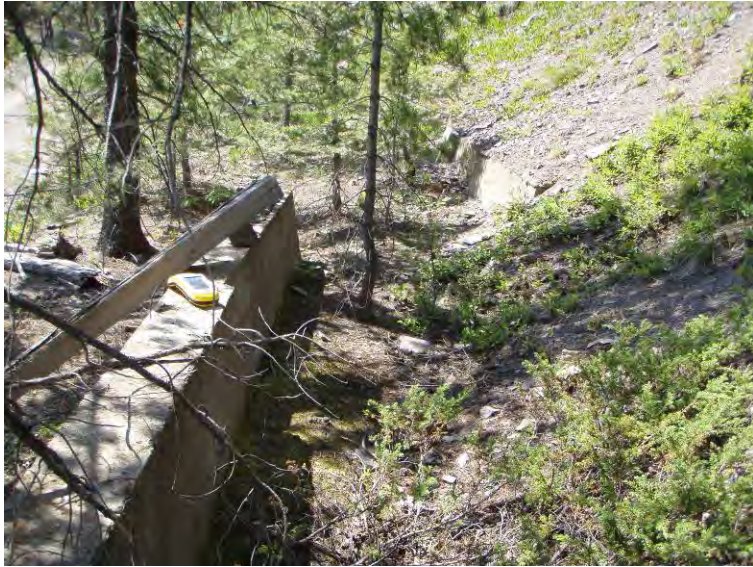
Photo 37: Retaining wall above Mike Horse town site & above Mike Horse Creek Road (looking SW).
