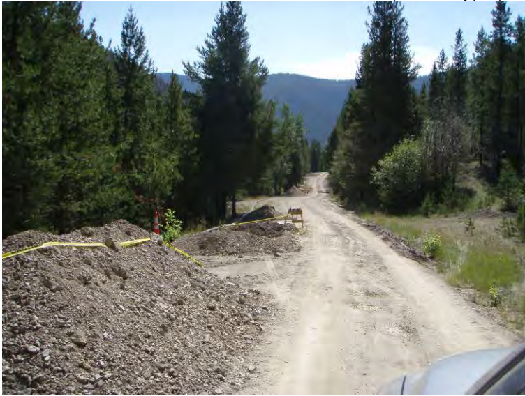
Photo 33: Pipeline repairs from Mike Horse adit to WTP on east side of Mike Horse Creek Road (looking S).
