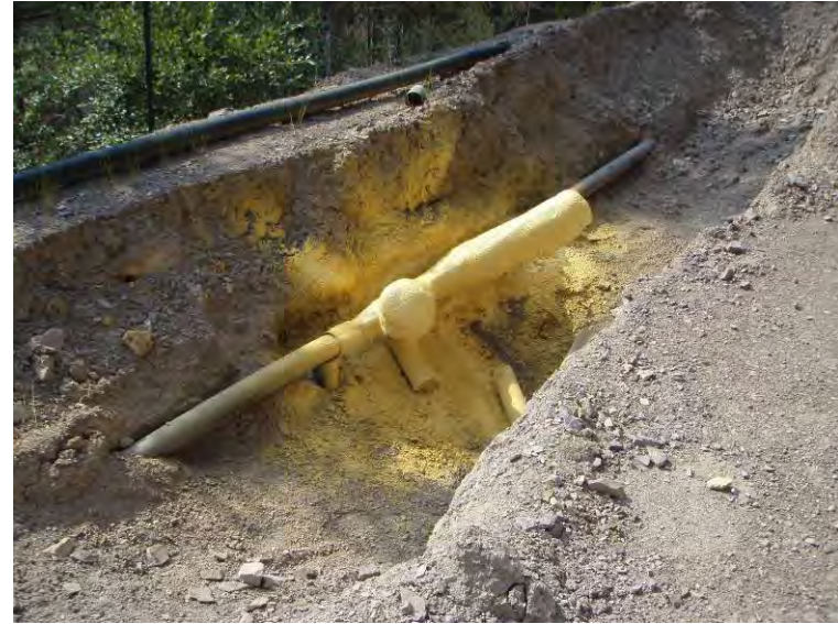
Photo 52: Mike Horse Creek Road repair pit & foam insulated pipe cleanouts (looking S-SW).
