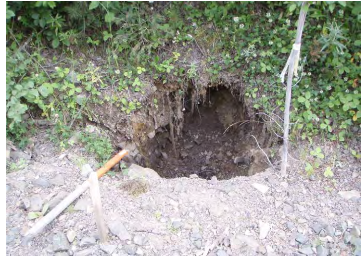
Photo 44: Subsidence of collapsed adit above the water treatment plant & underlying Mike Horse Creek Road (looking SW).
