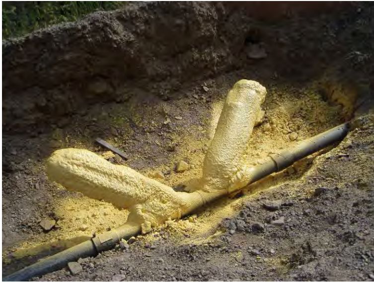
Photo 47: Mike Horse Creek Road repair pit & foam insulated pipe cleanouts (looking E).
