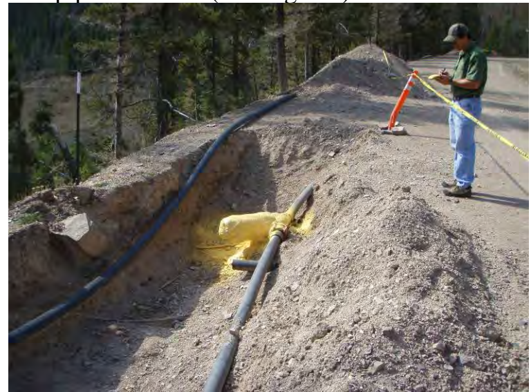
Photo 50: Mike Horse Creek Road repair pit & foam insulated pipe cleanouts (looking SW).
