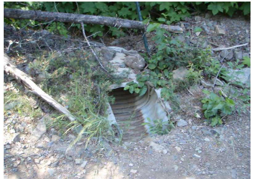
Photo 32: Damaged 24" CMP under Mike Horse Creek Road near the water treatment plant (looking NE).
