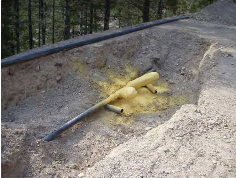
Photo 51: Mike Horse Creek Road repair pit & foam insulated pipe cleanouts (looking S).
