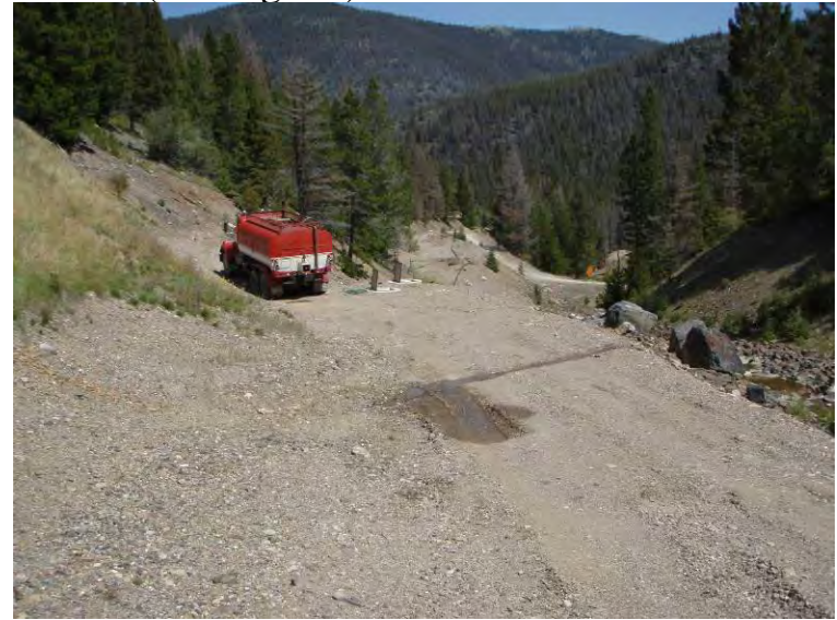
Photo 34: Seep in lower road to Mike Horse Mine and pipe work to WTP (looking NE).
