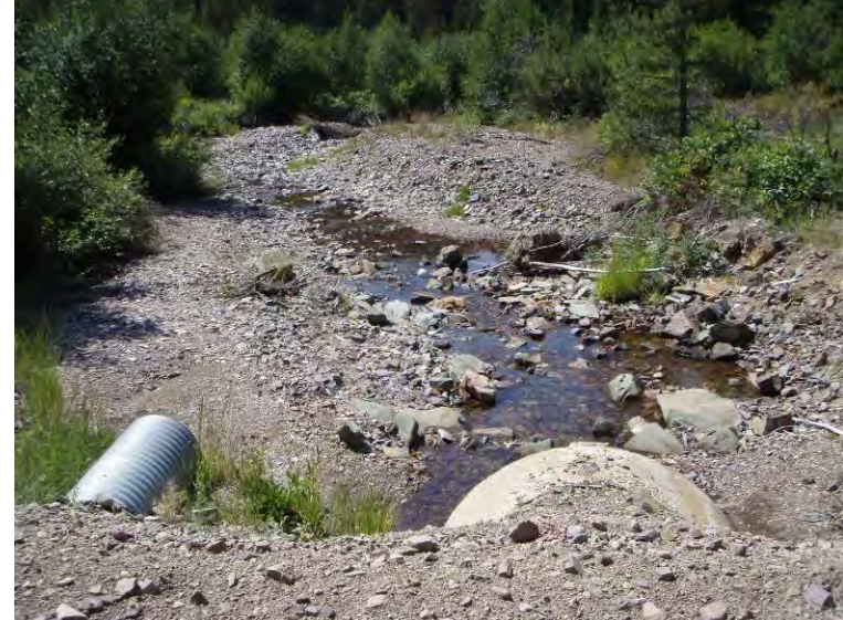
Photo 30: Shave Creek culverts in Mike Horse Creek Road 24" CMP and 54" RCP (looking SW).
