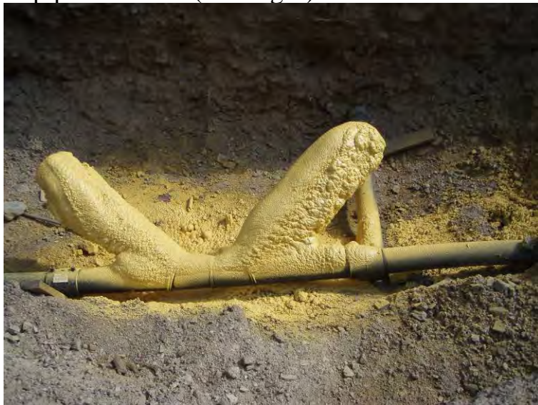
Photo 49: Mike Horse Creek Road repair pit & foam insulated pipe cleanouts (looking E).
