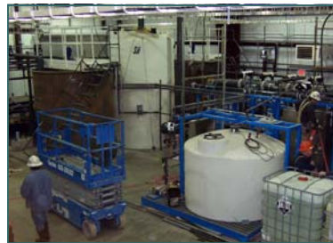
Water filtration system treats an average of 91,000 gallons a day.
