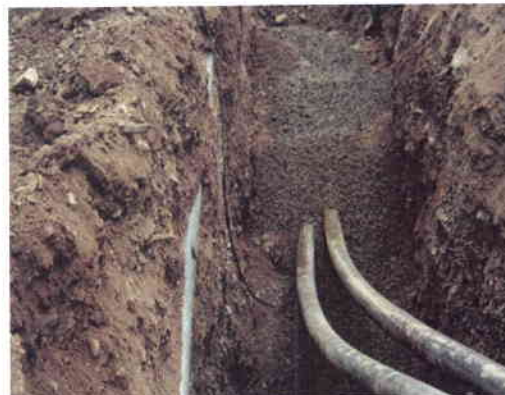
Replacement pipes for the Water Treatment Plant. Old thin-walled pipeline was buried approximately 2 feet below ground. The new pipes are at least 6 feet down.
