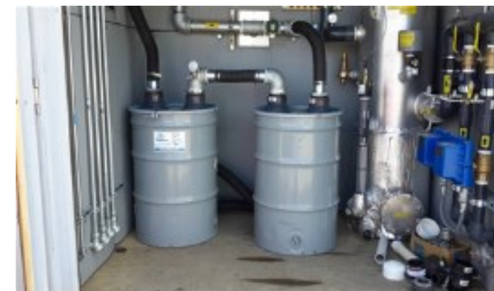
Inside the SVE equipment shed for the soil vapor extraction enhanced bioremediation system.
