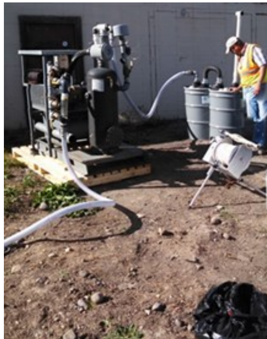
Horizontal SVE well testing
