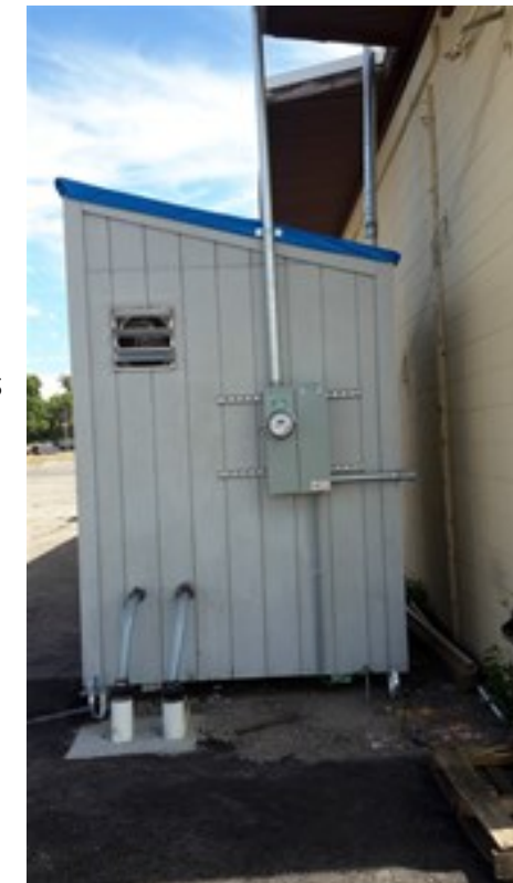
Equipment shed for the soil vapor extraction enhanced bioremediation system.
