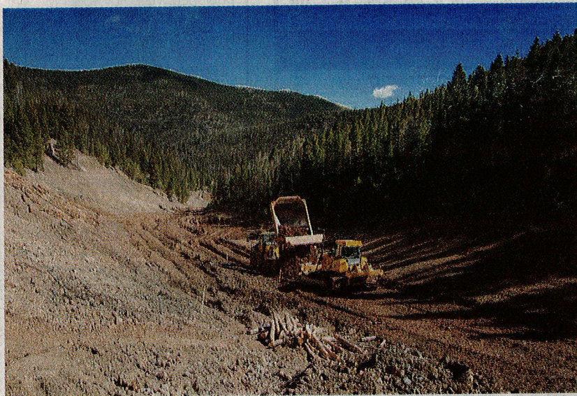
A dumptruck drops off a load of clean fill material in the Mike Horse Creek drainage as a bulldozer waits to spread it out to rebuild the creeks floodplain.
