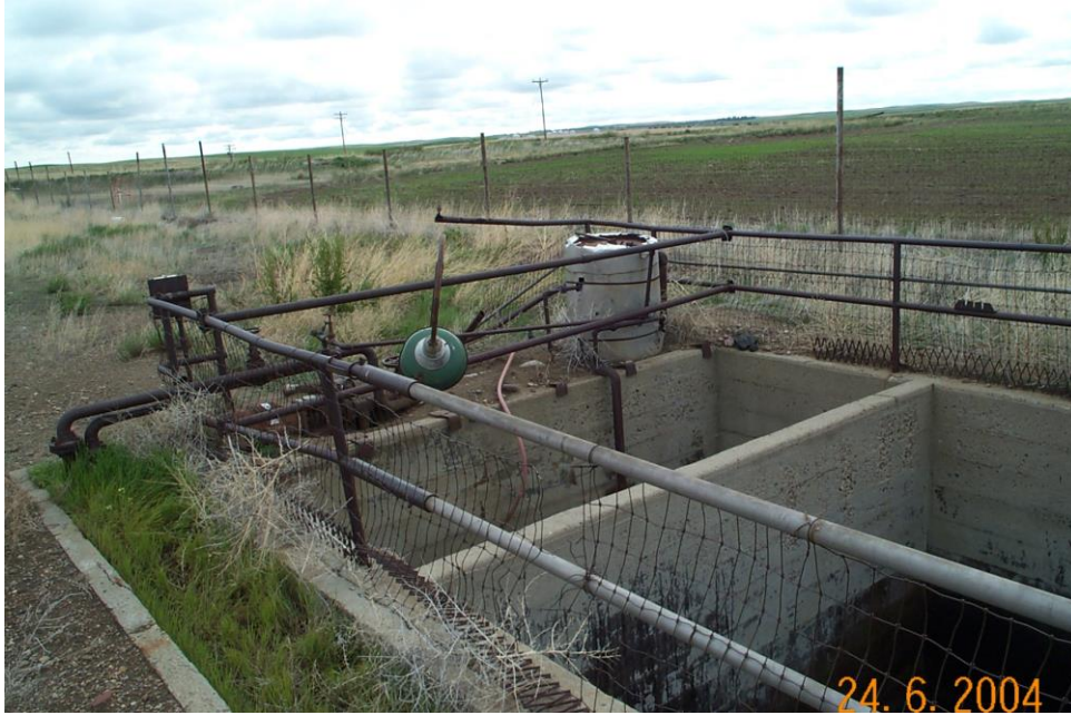
Old API Separator
