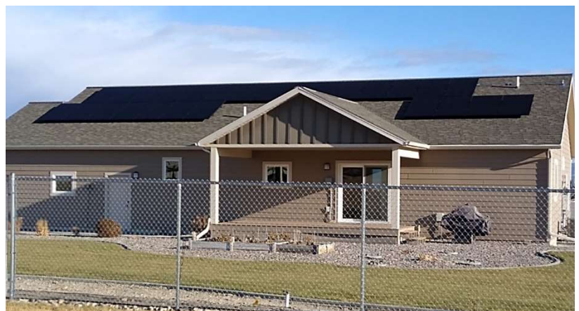
Montana Home with an 8.75 kW Solar PV System
