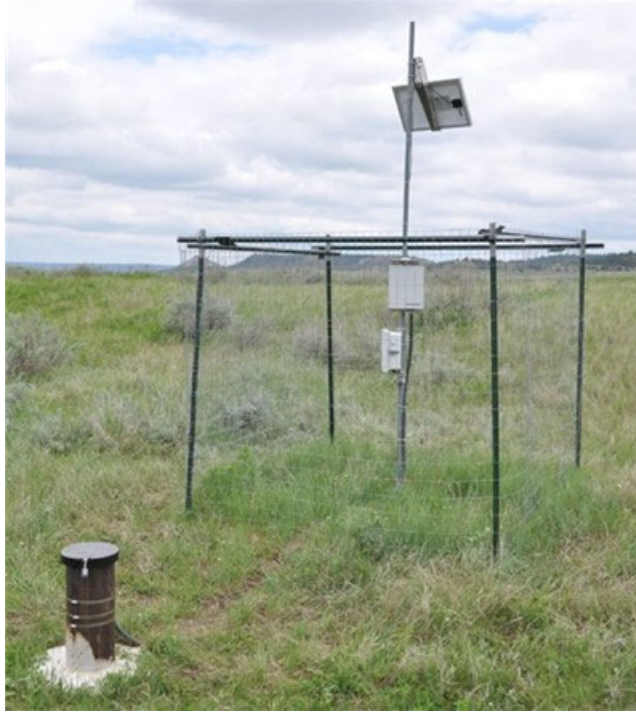
Figure 3.17. Well PW 736 with companion datalogger enclosure, solar panel, and fenced enclosure.
