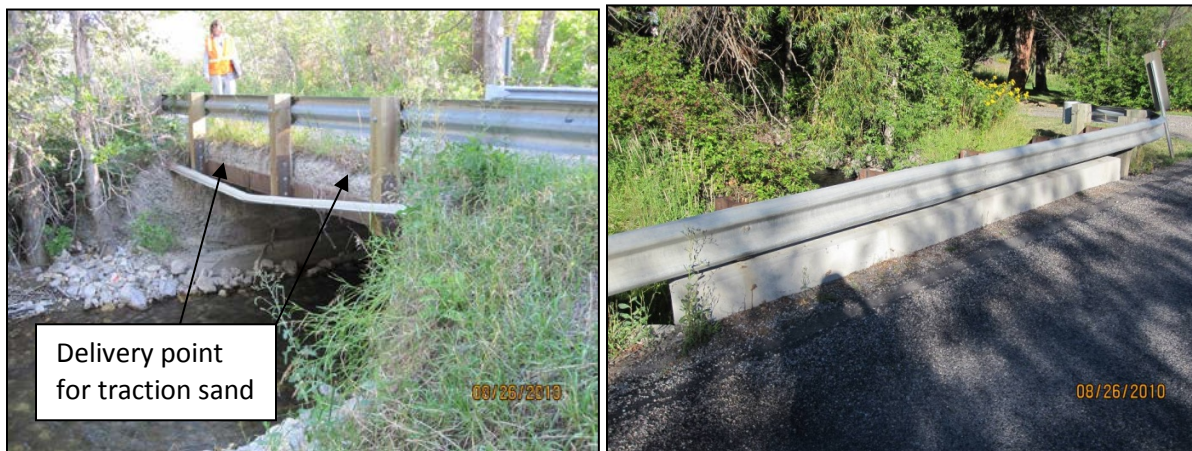
Figure 5-4. Crossing with observed areas of traction sand delivery (left); curbed crossing (right).
