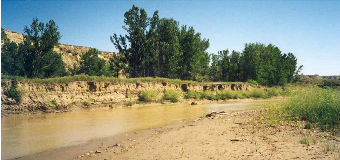
Figure 3-7. High banks along the Teton River are indicative of downcutting and restricted access to the flood plain (far bank in photo).
