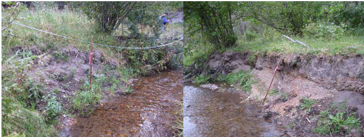
Figure 4-19. Typical eroding streambank conditions in Smart Creek Reach 13-01.
