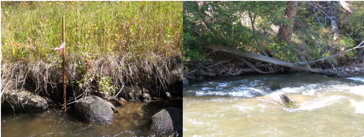
Figure 4-12. Typical eroding streambank conditions in Flint Creek Reach 11-04.
