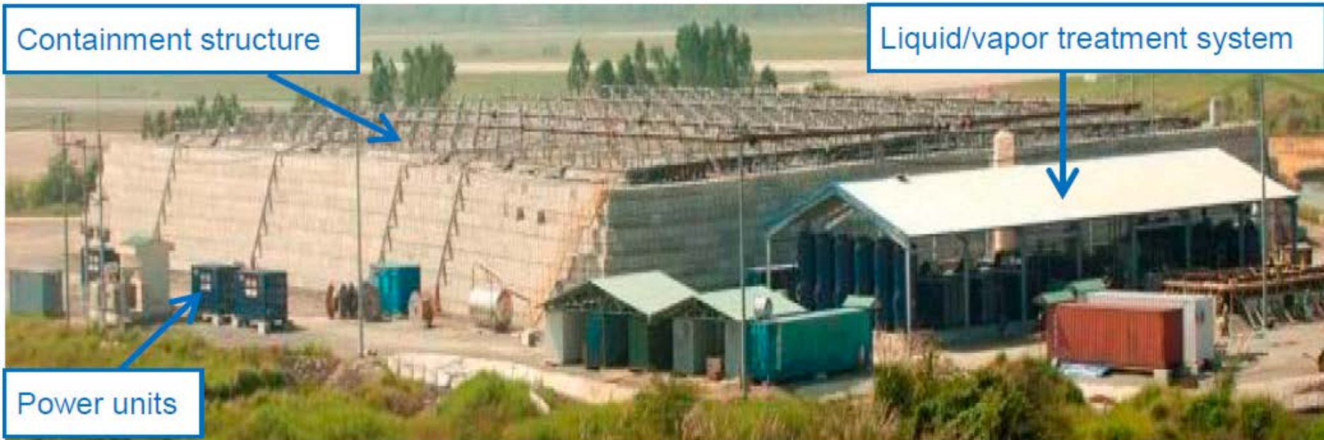
Containment structure and liquid/vapor treatment system
