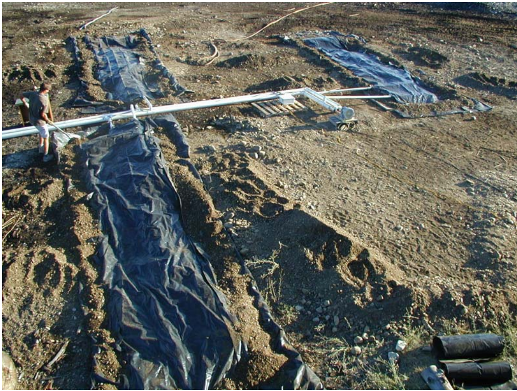
Figure 12. Biocells covered with polyethylene sheeting. Edges of sheeting were secured with soil.
