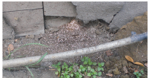
Vermiculite shown leaking from siding on the exterior of a structure
