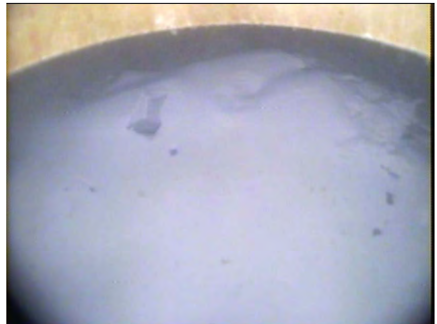
Photo of white precipitate accumulated at bottom of well (210 feet). Lower edge of PVC casing that is visible at top of photo shows no scale at this depth.
