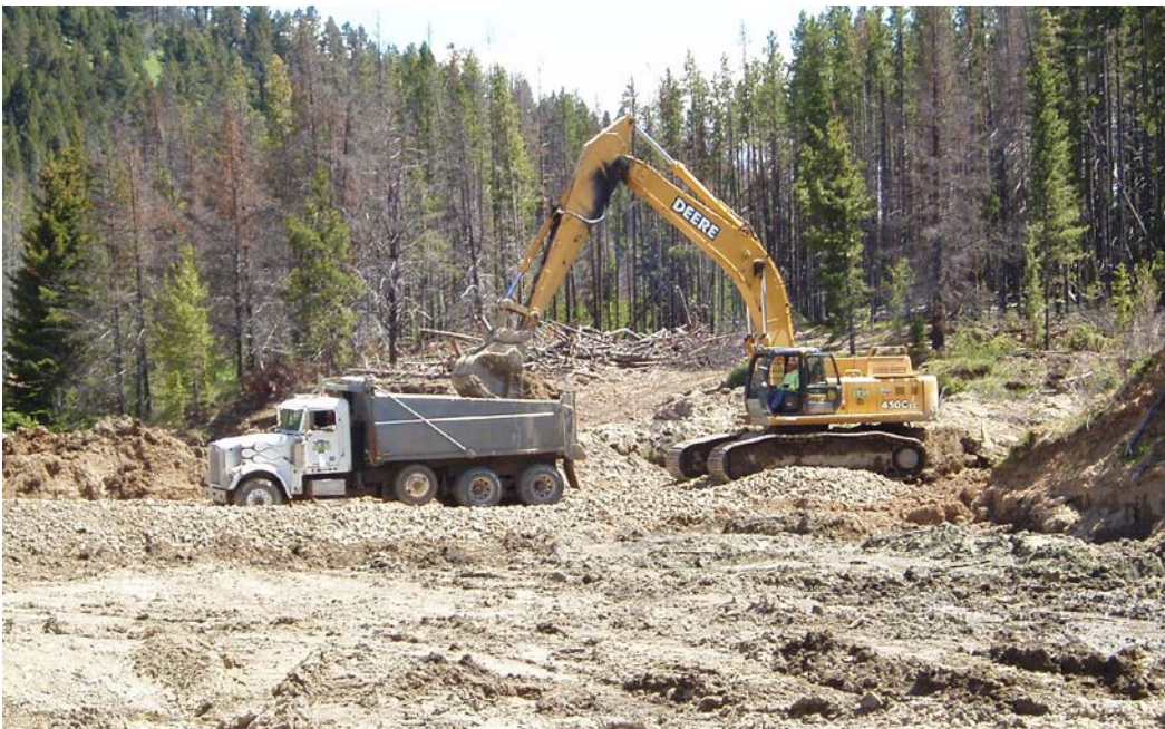
Figure 2. Excavation of tailings from the Bald Butte Mill in the Dog Creek drainage.
