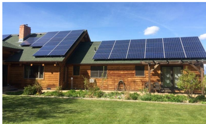
Figure 6: A residential solar electric array in Bozeman funded by the AERLP in FY16.
