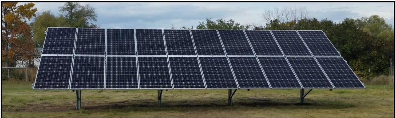
FY17-funded, ground-mounted solar array in Hamilton
