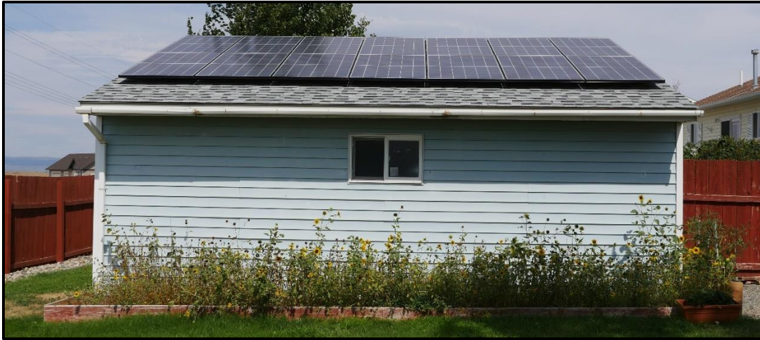
FY18-funded, rooftop solar array in East Helena
