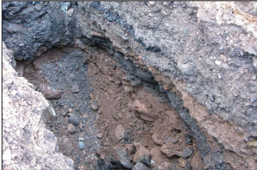
Petroleum-impacted soil observed in test pit at TB008 (Vat Area).
