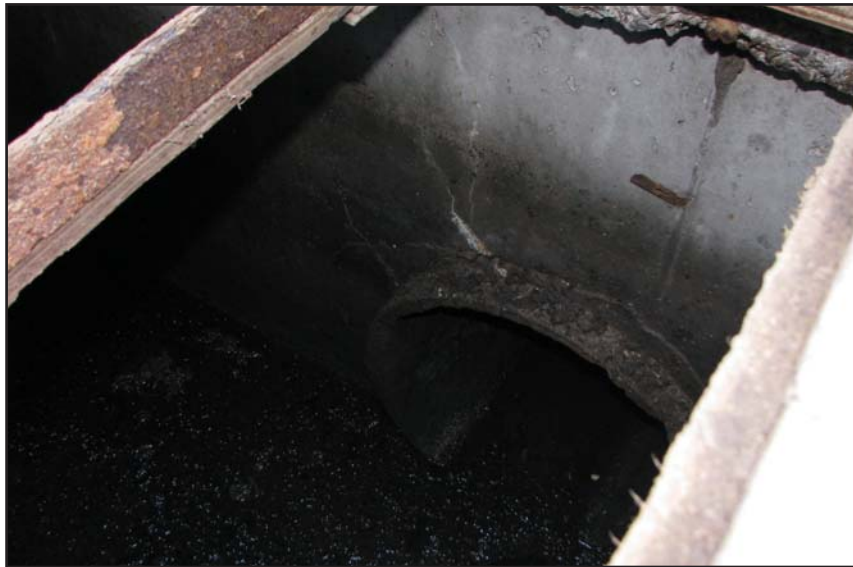
Glue/resin wastewater tank interior.
